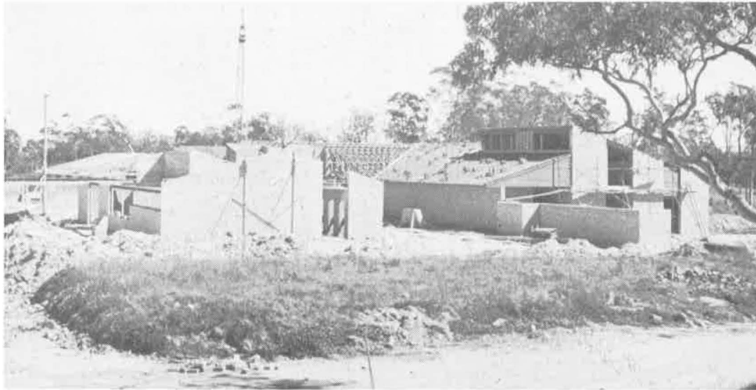
Construction is well under way on Stage I of the Wyong Hospital at Kanwal.
